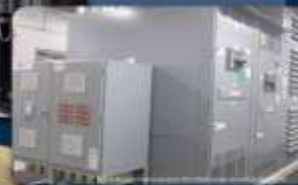
Fire & Gas Suppression Systems
