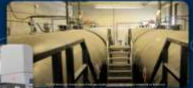
Generators; Storage for Fuel, Water
